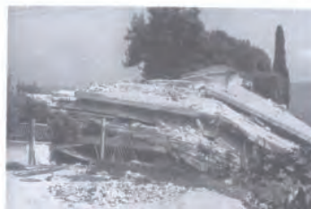
Figure 19 - Collapse of a 4-story reinforced concrete apartment building. Severely damaged by the main shock, the building collapsed in a minor aftershock on 9-14-1986.
