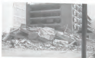
Figure 16 - Collapse of a 3-story reinforced concrete apartment building on pilotis. Severely damaged by the main shock, the building collapsed in the major aftershock of 9-15-1986.
