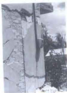
Photo 9, 10: Total collapse of category B building in the village of Kentro (top) and total failure of a shear wall of a two-storey building in Eani (bottom).
