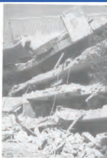
Figure 15 - Collapse of a 3-story reinforced concrete apartment building on pilotis. The building collapsed in the main shock killing 6 people. 19 people were rescued.
